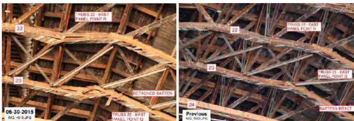
Figure 2. Truss damage progress at Trusses 22 and 23 East near Panel Points R and Q.
