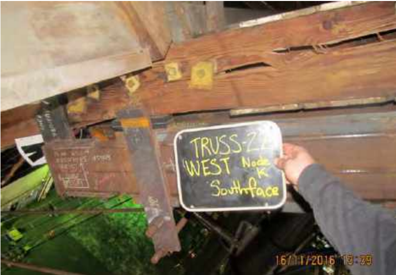
Chord damage at node K after exoskeleton install
